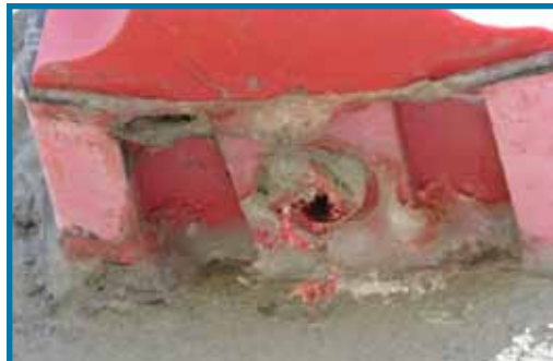
Silicone caulk has been used improperly between the product and the gasket. A weep hole has been drilled into the bottom conduit plug. Drilling holes into the bottom conduit plug is not recommended.
