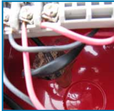
A conduit connector has not been used to run wiring into the back opening. This provides a path for water to enter the device.
