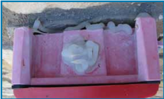
Silicone caulk has been used improperly in place of a conduit plug. Silicone caulk has not been appropriately applied to seal the space between the rough wall surface and the back box.
