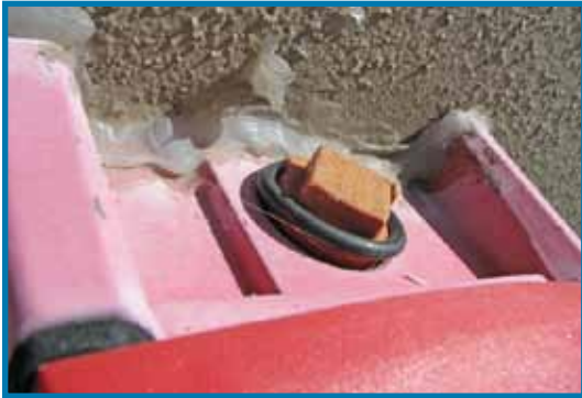
This gasket has been installed incorrectly, resting on top of the conduit plug rather than being compressed between the plug and the back box.
